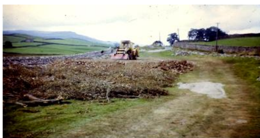
Towards Hawes; trees felled to make way for the new road, being used to support it over a boggy section
